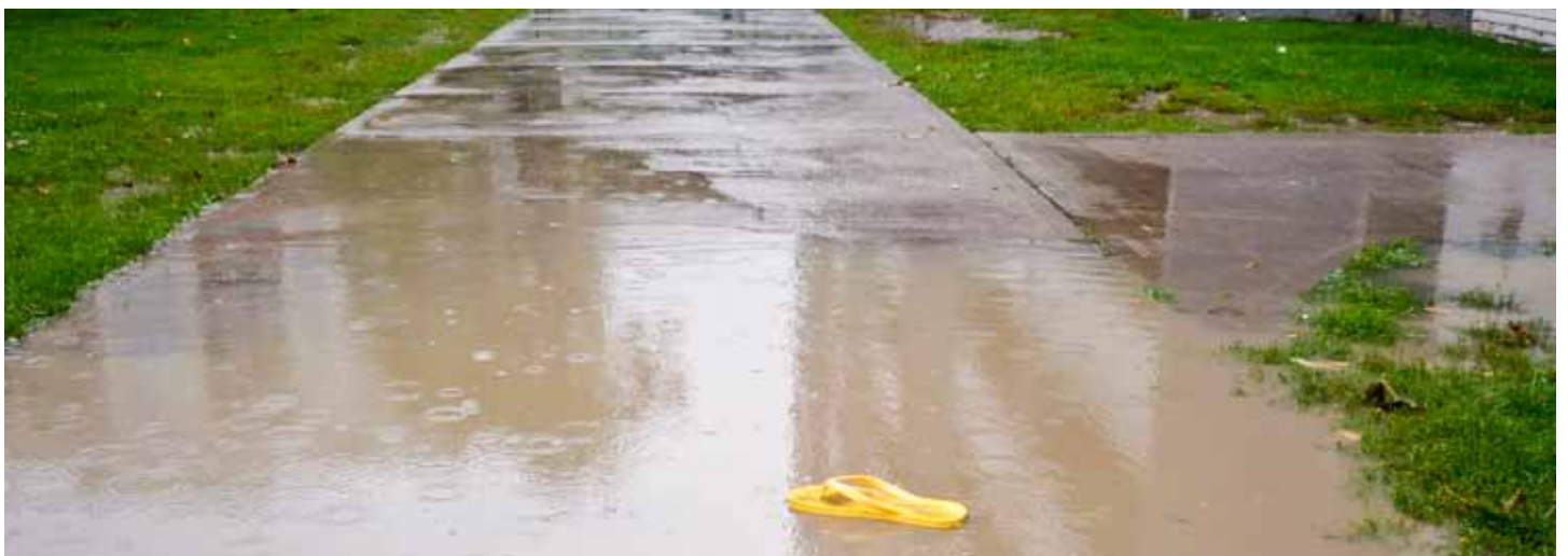
Pooling water on a path in St James Town
